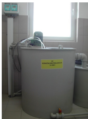
(a) Final neutralization tank.
