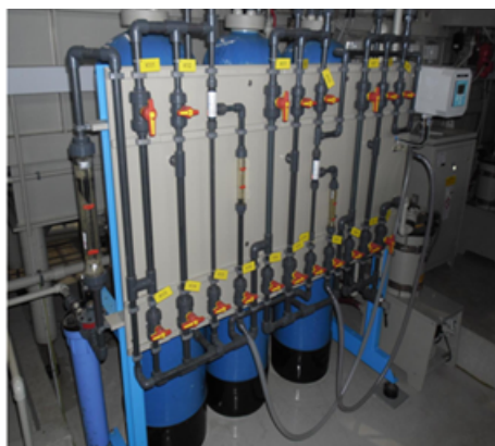
(a) Cation and two anionic JI-columns 1 with pipe distribution with valves, injectors, H 2 O flow meters and regeneration agents, pressure gauge, conductometer and cartridge filter on the support structure for CN - -washed water.
