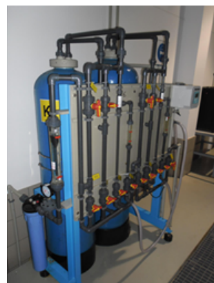
(b) Cation and anion JI-columns 2 with pipe distribution with valves, injectors, H 2 O flow meters and regeneration agents, pressure gauge, conductometer and cartridge filter on the support structure for rinse water without CN - .
