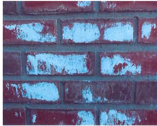
Figure 2. Typical white efflorescent salts on masonry
